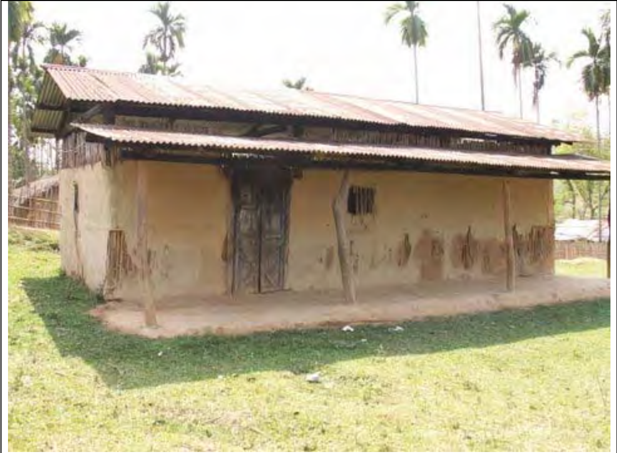
Photo 3: Dikchak Pre-Primary School – Current building is in urgent need of repair or replacement
