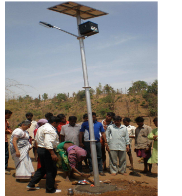
Dr. Sujit, Mrs. Patwardhan and local residents during solar street lamp installation
